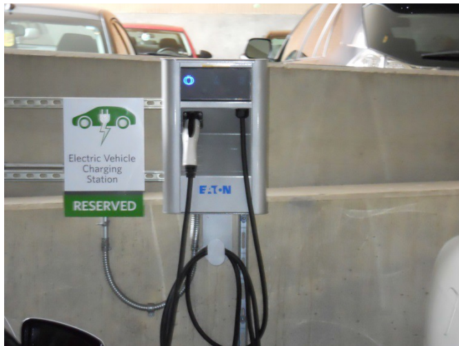
Figure 34. Installed electric vehicle charging station
